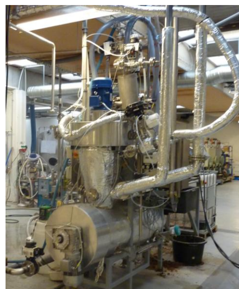
Continuous pretreatment facility. Operates with capacity of up to 50 kg per hour at BioGasol (Ballerup, Denmark).
